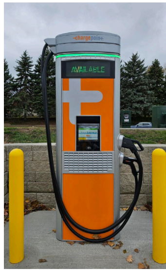
ChargePoint Express Level 3 DC Fast Charger
